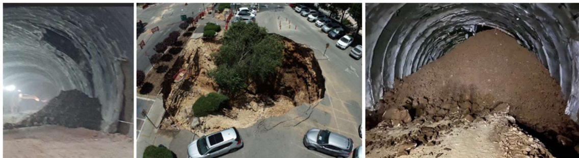
Figure 2. Onset of the TU4 collapse (left), formation of the surface crater (center – approximately 20 m diameter) and debris material inside the tunnel (property of the authors).
